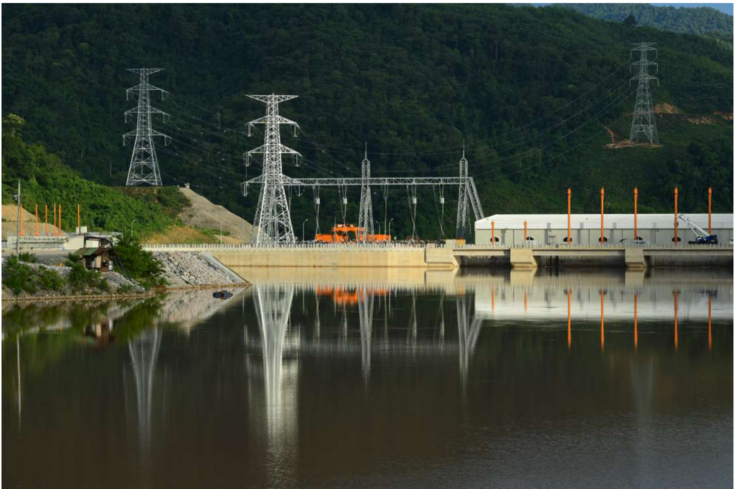
500 kV Takeoff yard and Transmission towers
